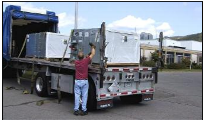
New AC/Heating units for the O/R, Physical Therapy, and Cardiology sections being delivered to the Hospital September 2 nd .
