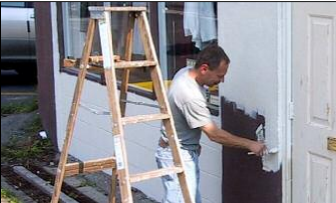
Left: Marc Kalipolites puts some fresh paint on his Rte.209 storefront, one of the many individual efforts sprucing up the Village.
